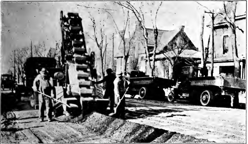
REMOVING EXCESS MATERIAL AFTER SCARIFYING AND RESHAPING MACADAM STREET IN DENVER PRIOR TO APPLICATION OF SHEET ASPHALT TOP
